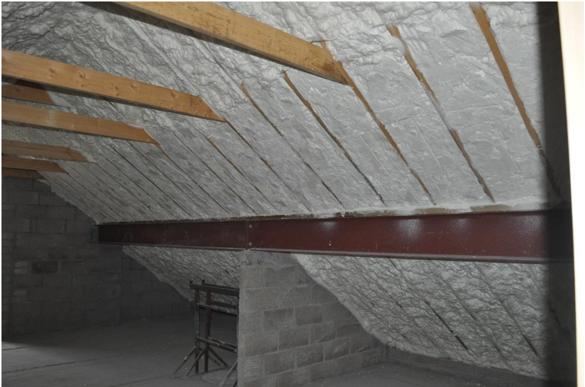
Figure 2 - close-up showing the Product detailing around steel RSJ and dwarf partition wall; prior to dressing back flush with the rafters
